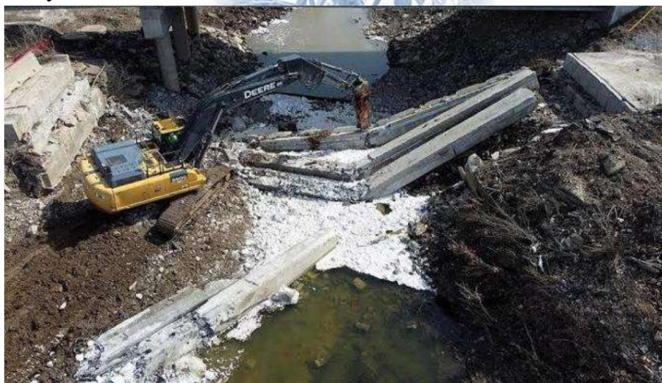
Figure 1. Technogenic Disturbance of Soil Layers at a Bridge Construction Site and Disposal of Construction Waste into the River Channel
